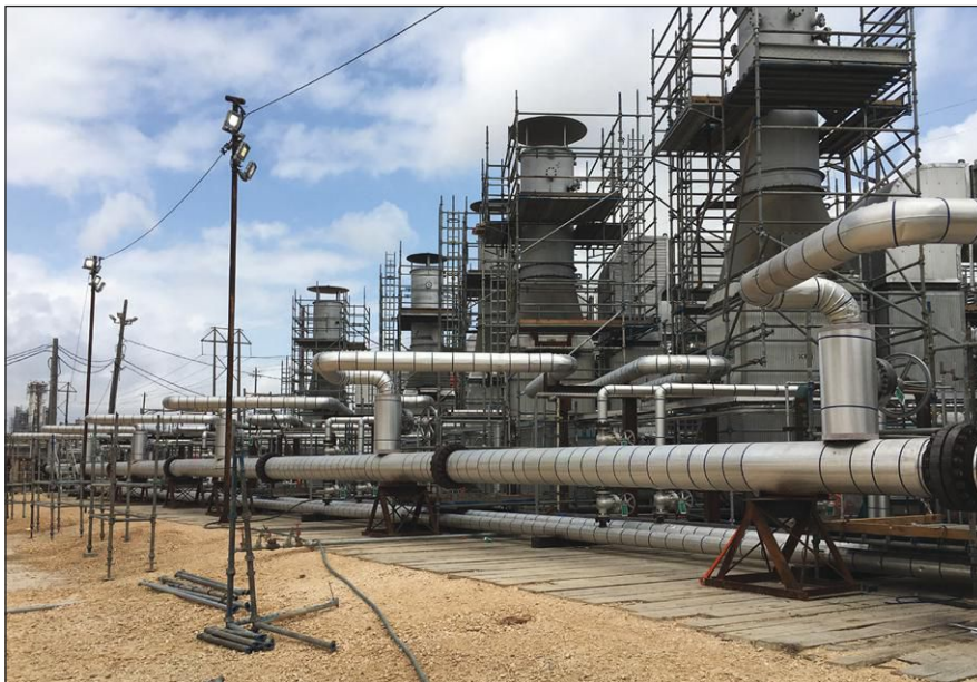
Figure 3: The temporary boiler equipment supplied process steam to meet facility demand for more than three years and was also instrumental in returning this facility to an operable state after the “Big Texas Freeze of 2021.”
